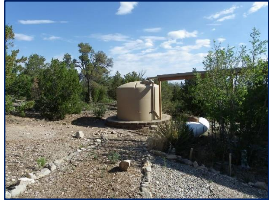
District Funded Water Harvesting Project
